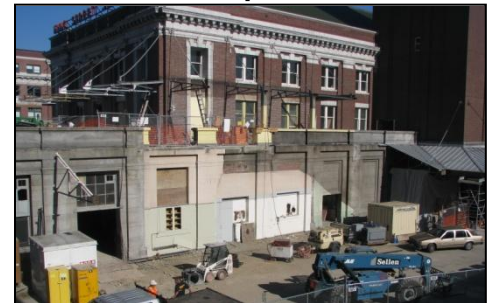
Above, the enclosure for the stairs and escalators to Jackson St. has been removed, along with the stairs and escalators. This was not a part of the original station. The open stairway build as part of the original building will be restored.
